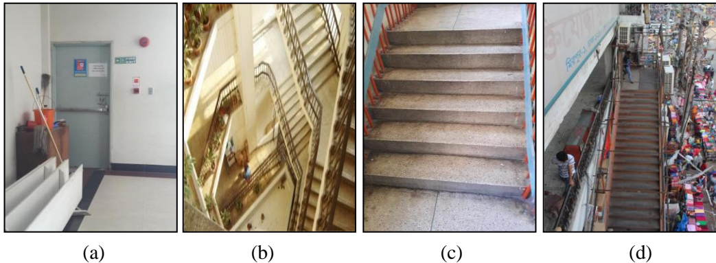
Fig. 3: (a) Locked emergency gate in Bashundhara City Shopping Mall, (b) Open stair will be a carrier of fire and smoke in Eastern Plaza, (c) Sloppy and narrow emergency stairs in Motalib Plaza and (d) Narrow and weak steel frame emergency stair in Muktijoddha Super Market
