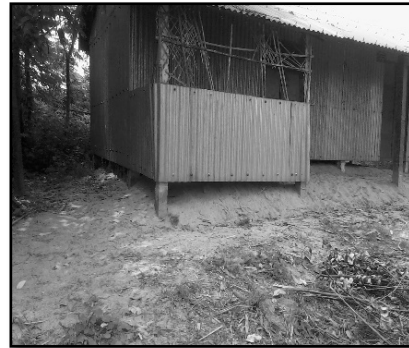
Fig 5: Housing deteriorating due to sandy soil at Shalhati Cluster village
